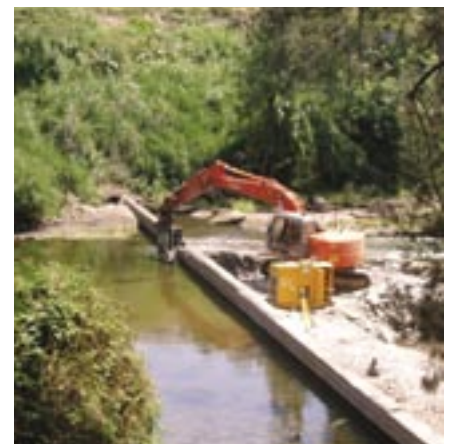
The Norco Weir at Casino restricted fish migration up and down stream. It was removed in 2007.
