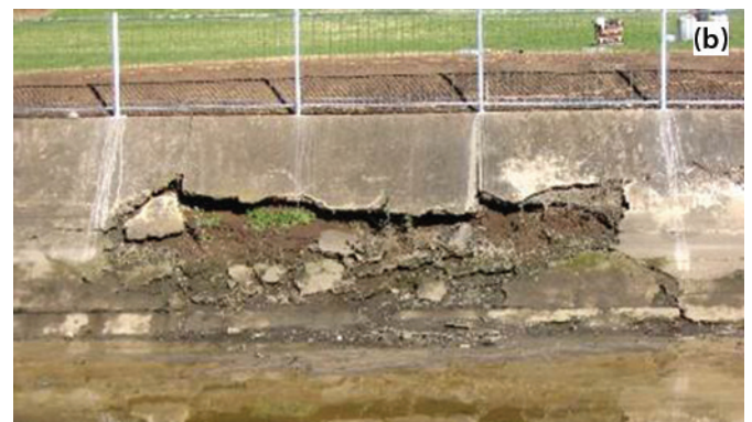
Figure 2. a) Burwood RH concrete bank with bottlebrush growing in cracks; b) Deteriorating section of concrete channel identified for renewal.
