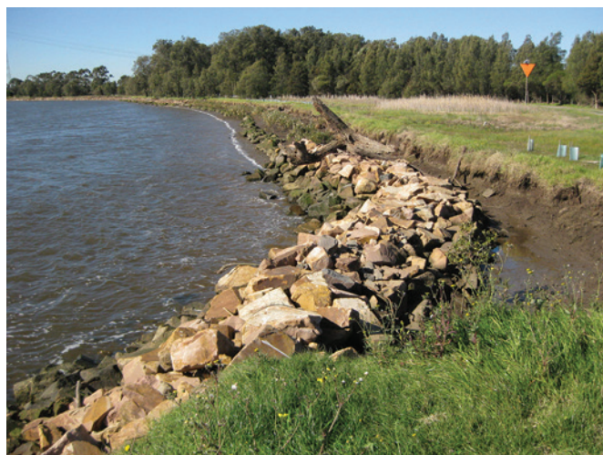
b) Photo point 4 post works July 2011, showing full scale rock fillet in foreground, low fillets beyond.
