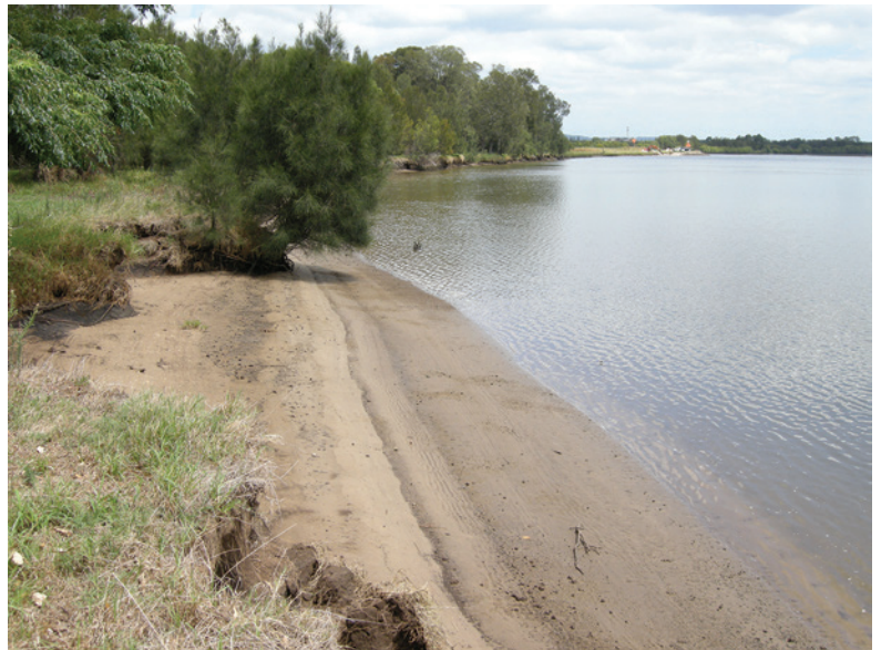
Figure 7. a) Photo point 10, highly undercut eroding bank before works, 2011.
