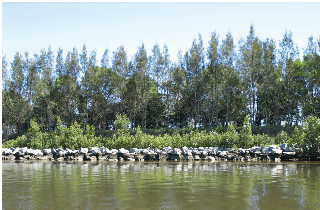
Figure 3. Rock fillet erosion control at Dumaresq Island, Manning Estuary showing supported mangrove growth.
