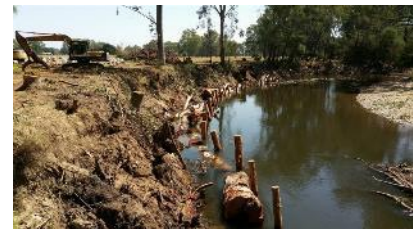
The placement of timber and rocks for erosion control and fish habitat will be complemented by riparian revegetation. Photo: North-east Catchment Management Authority.
