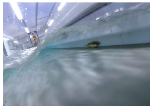
A Crimson-spotted rainbowfish navigates the fast flow by swimming in the slower water under the beam. A square beam installed along the length of a culvert wall can be incorporated into new structures and or retrofitted into existing culverts. Photo: Harriet Goodrich.
