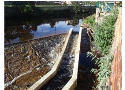
One of the fishways ('fish passes') that is enabling Salmon to find their way upstream in the River Don. Photo: Don Catchment Rivers Trust.
