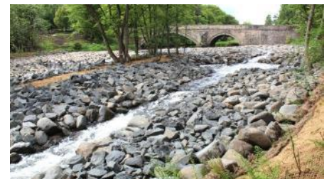
The rock ramp means fish, including Atlantic Salmon, can access spawning areas upstream. Photo: Forth Rivers Trust.
