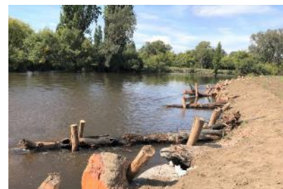
Bushfires rendered these trees burnt and dangerous however they make great snags and will help stabilise the riverbank. Photo: Murray Local Land Services.
