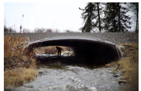
Lake Orbin contained a lot of juvenile Coho Salmon and during the very hot summer they were suffocating, stressed out by a lack of oxygen and hot water temperatures. Once the flow was re-established, the juvenile fish just barrelled up through the culvert and into the cool groundwater fed stream. Photo: USFWS/Katrina Liebich.
