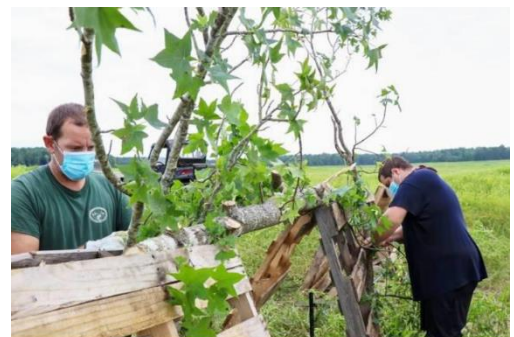
The advantage of installing fish habitat in a drained lake – building fish cribs in-situ. Photo: Special to The Commercial.
