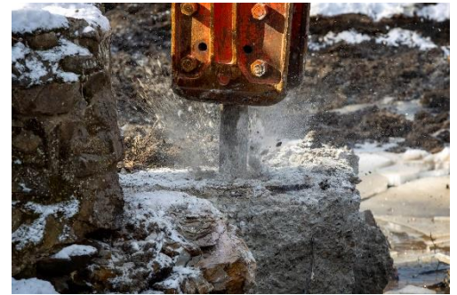
Heavy machinery made short work of removing one of over 1000 dams and weirs that impacting fish passage. Photo: Robin Lubbock/WBUR.
