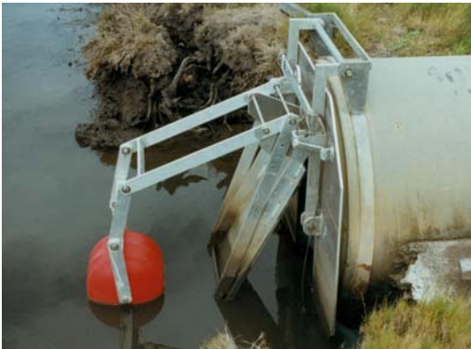
A simple float on a tidal floodgate allows water to flow and fish to pass through the gate with the rise and fall of the tide. Images I&I NSW.
