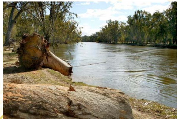
Photo 3: Logs are dragged to the desired position in the River with the 'cable dragging technique'. Photo: Michael Bell
