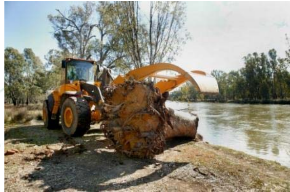
Photo 1: Logs are placed into position on the river bank. Photo: Michael Bell
