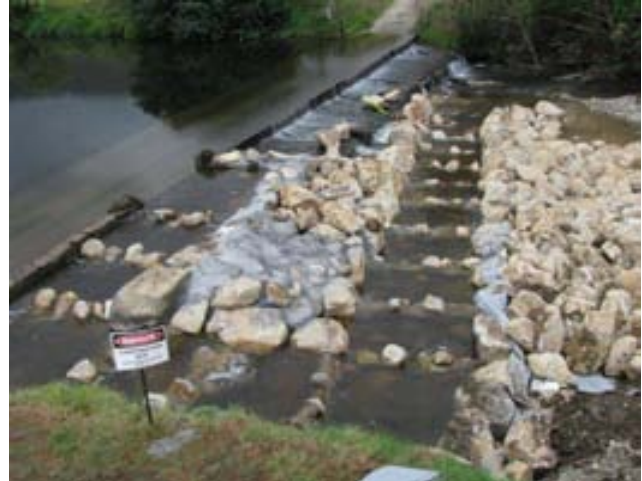
Partial width rockramp at Hawdons Crossing on Gloucester River. Photo: Shaun Morris
