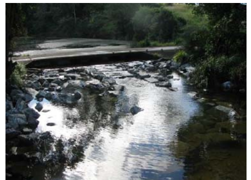
The Dargavilles Crossing fishway links important estuarine and freshwater aquatic habitat areas of the Wallamba River.
