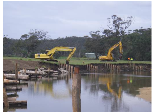
Construction of timber groynes along the Murrumbidgee River have contributed to improvements in fish habitat. Image: Southern Rivers CMA
