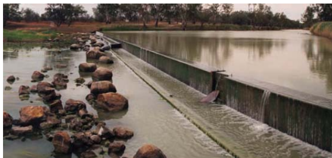
The Brewarrina weir. The existing fishway is inadequate and work is now underway to improve passage for native fish. Photo: David Cordina
