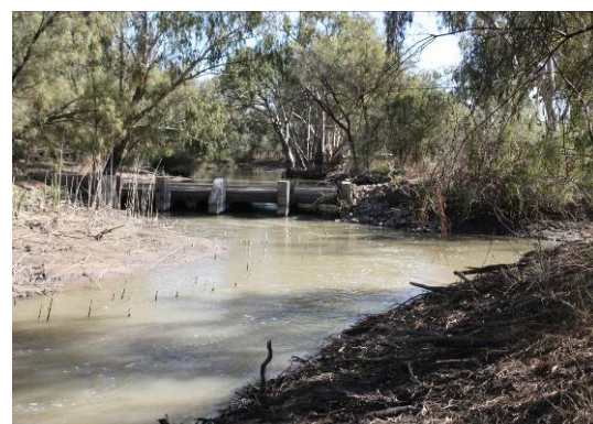
The current structure viewed from upstream. The structure was partially remediated by taking out the drop boards and removing a sill that created a 20cm drop (native fish are hindered by a drop of as little as 10cm). Further remediation is now being undertaken to reduce the velocity of flow, which has also been identified as hindering the passage of native fish at this site. Photo: Rodney Price.
