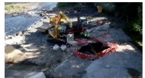
The start of the construction of the Hexham Bridge fishway. Photo: Tyne River Trust
