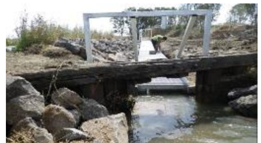
The new fishway on the Barwon River barrage. Image: D. Lovric (extracted from report)
