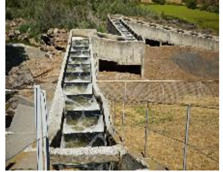
Built to 1950's standards, the removal of this fish ladder, and the dam it serves, will benefit fish. Photo: Kevin N. Hume.
