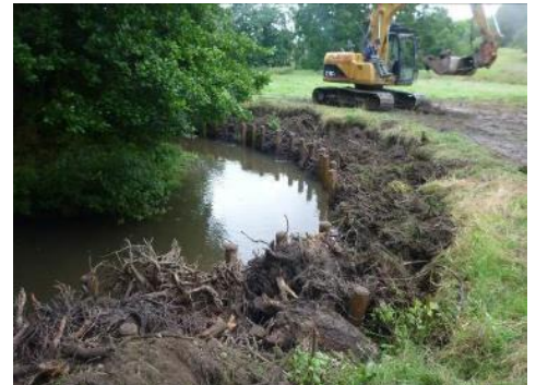
Root plates from alder trees were used to protect the outside of a meander bend. These will promote bed scour and deepening of the pool, making it more suitable for larger trout. Photo: Wild Trout Trust.
