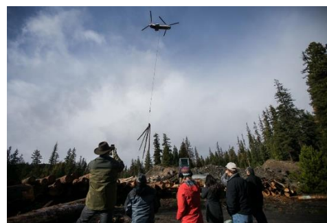
Helicopters were the most cost-effective option for moving the logs and avoided the significant damage to roads likely if trucks had been used. Photo: Amanda Ray, Yakima Herald-Republic.
