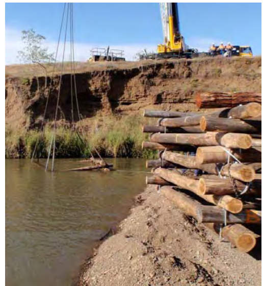
Once built, the fish hotels were lifted into place through the use of a crane, and are held in place by driven piles and large rocks. Photo: M. Elsley
